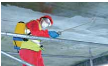
Principle 11, method 11.3 Corrosion at the cathodic areas of the reinforcement is inhibited by the use of Protectosil CIT.
